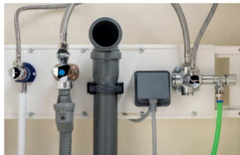
Cleanly and clearly mounted: cold and hot water, sink drain, surface-mounted socket, connection for drinking water pipe (e.g. for a coffee machine with a fixed water connection or a refrigerator with an ice cube make).
